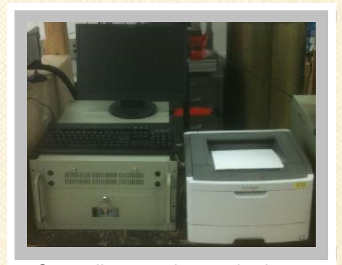
Controller, monitor and printer
